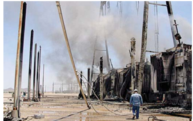
FIGURE 10 | Westwing Substation. Five Transformers Were Damaged in a July 4, 2006 Fire in Northwest Phoenix
