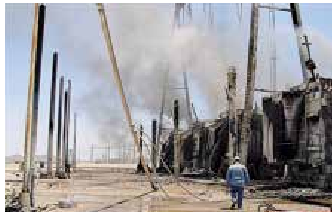
FIGURE 10 | Westwing Substation. Five Transformers Were Damaged in a July 4, 2006 Fire in Northwest Phoenix
