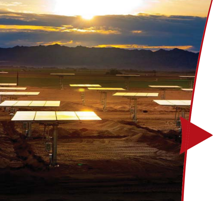
Solar array, Arizona Western College.
